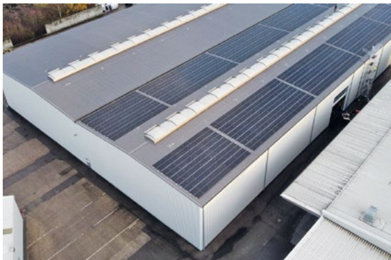
Photovoltaic system installed at the Lauingen site in 2022. Photo: Innolation GmbH, Lauingen, DE
