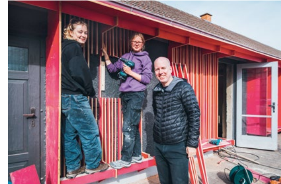
Seventy specialist tradespeople and students are involved in the IBA Sundhausen international building exhibition project – and they are supported by international partners. The Technical University Berlin, the Veldacademie with the Technical University Delft, the Technical University Vienna, PUC Santiago de Chile, the Bauhaus-Universität Weimar, and vocational schools for painters across the whole of Germany want to make rural living more attractive. The aim is to offer a changing programme of health care services and create a venue for events.
