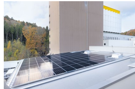
Photovoltaic systems installed at the Stühlingen site in 2022 (2/2). Photo: Sto SE & Co. KGaA, Stühlingen, DE
