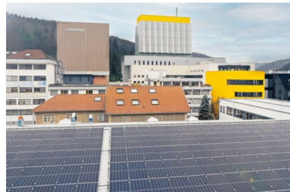
Photovoltaic systems installed at the Stühlingen site in 2022 (1/2). Photo: Sto SE & Co. KGaA, Stühlingen, DE
